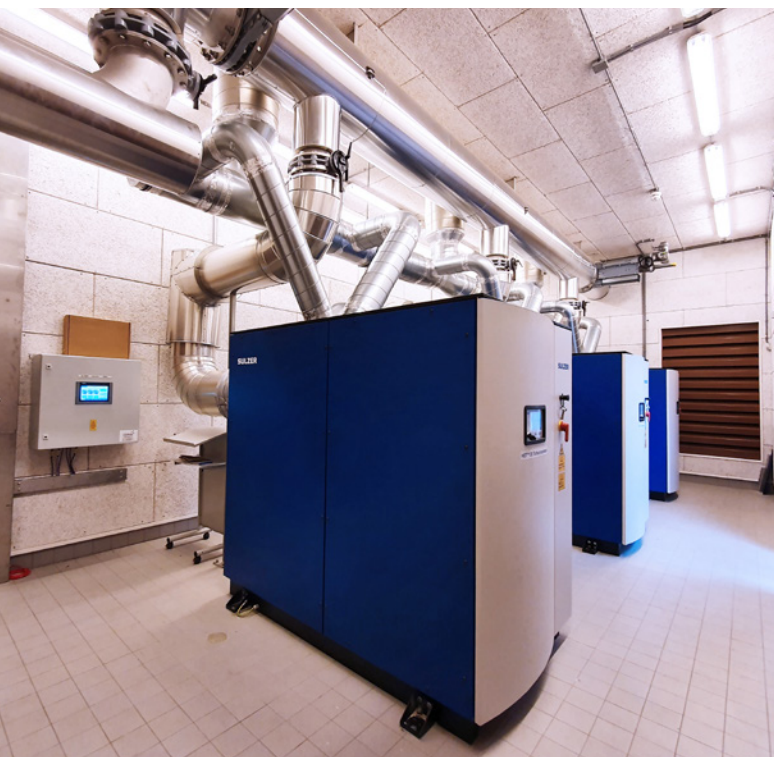
Photo 2: This is the new setup for the blower room shown in photo 1. A suitable set of HST 20 blowers could be determined to meet the need and by appropriately adapting the pipework could be made to fit the existing blower room.
