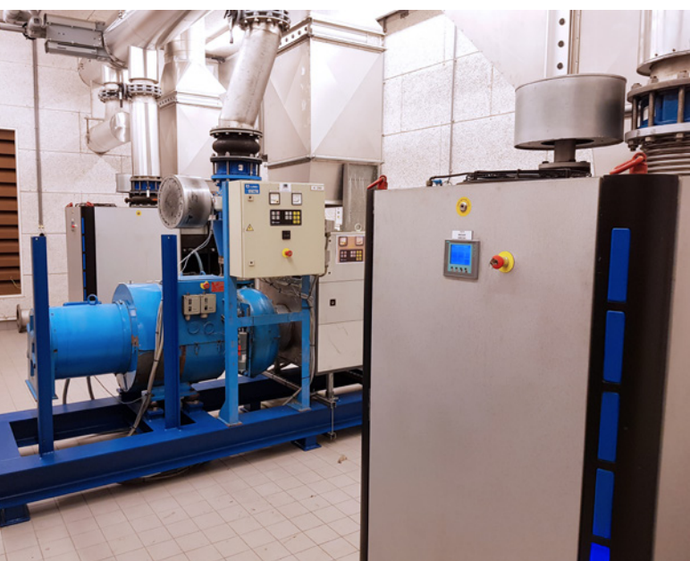
Photo 1: Before: The air foil bearing blowers at this site had technical issues and a rental centrifugal blower was supporting the operation
