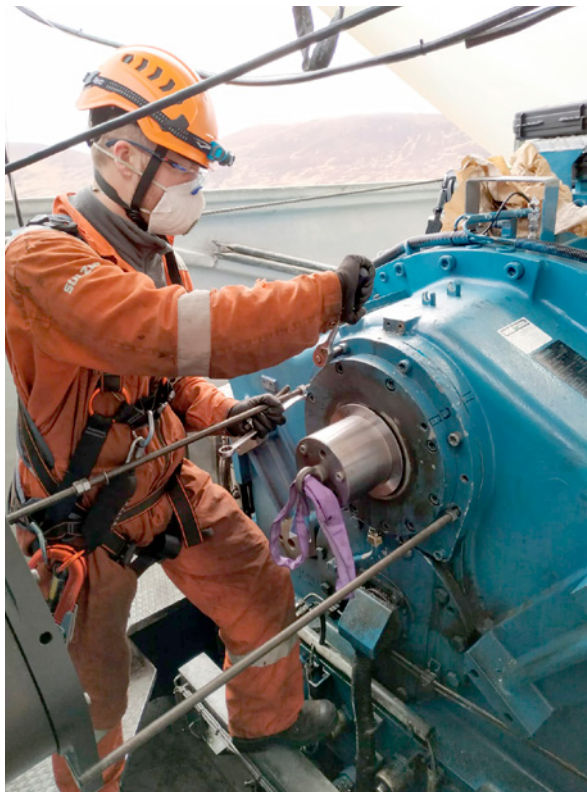
Sulzer delivers maintenance services for almost all components in the nacelle
