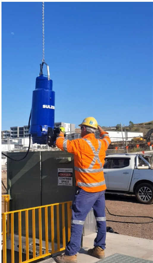
The new pumping station was equipped with Sulzer pumps and a grinder.
