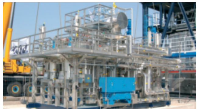
Skid mounted unit for MDI at Huntsman in the Netherlands
