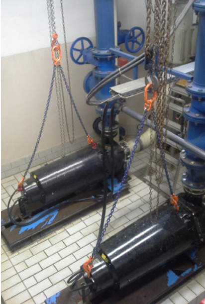
Submersible sewage pumps type ABS XFP installed in the pumping station
