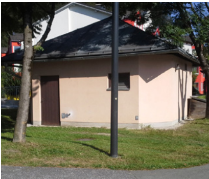
Network pumping station in Zell am See
