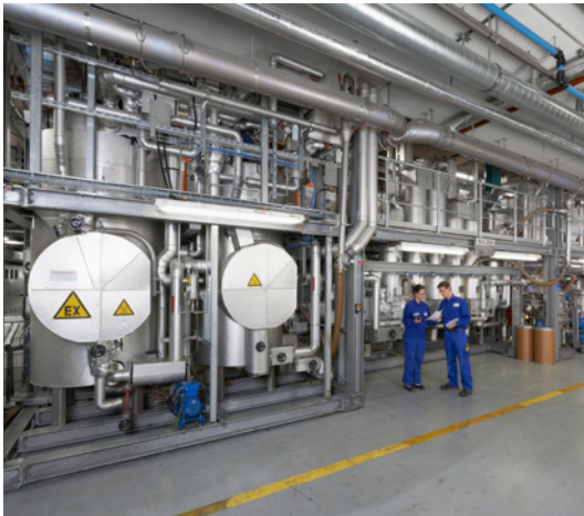
PLA biopolymer pilot plant built by Sulzer
