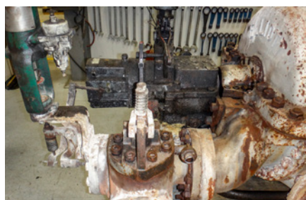
Rebuild governor and trip unit. Replace linkage bushings.
