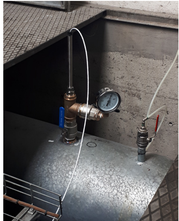
Flow and pressure data can support an energy audit and the process of raising capital for improvements.
