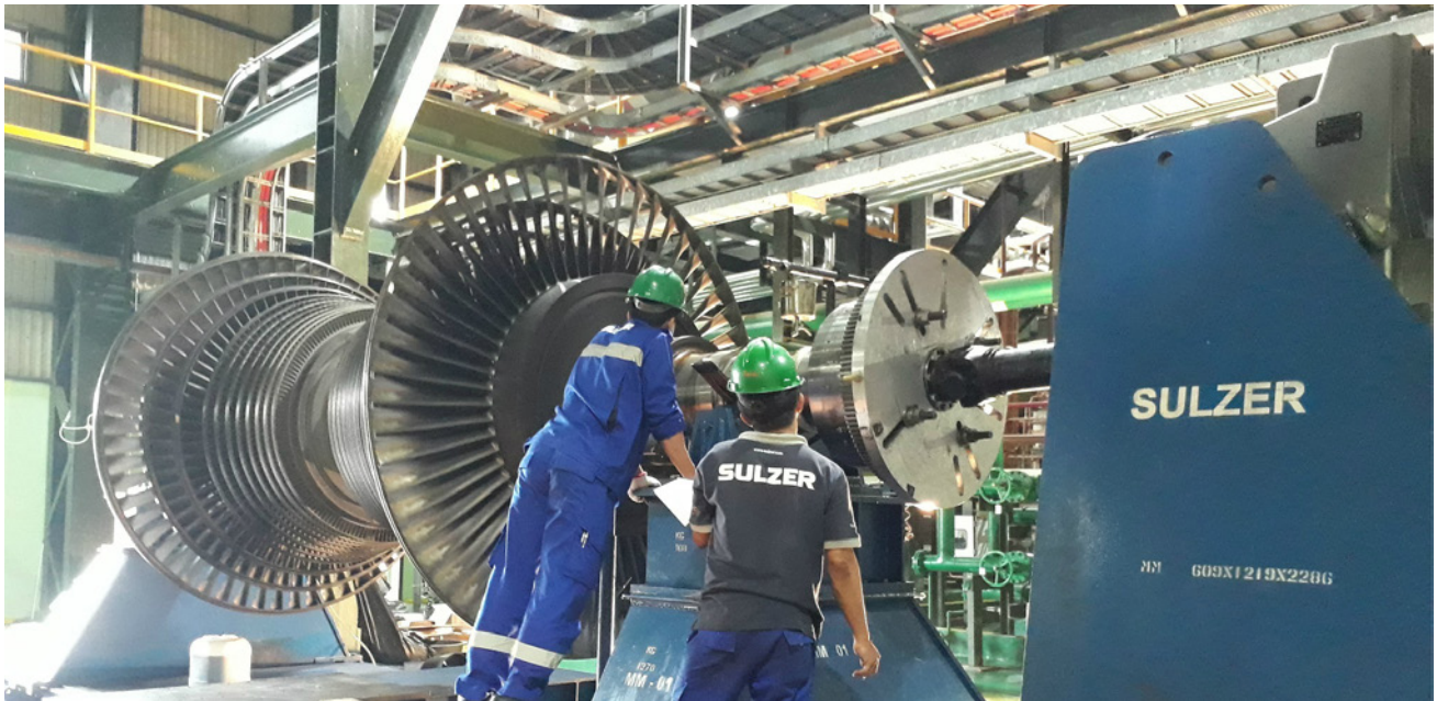
The turbine rotor was installed on the mobile lathe for inspection and repair
