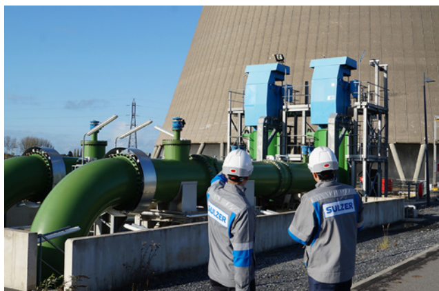
Sulzer experts from France and Switzerland worked to propose a solution that met EDF's technical requirements.
