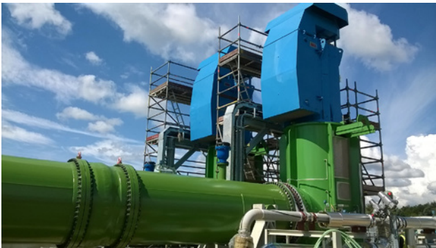
Installation of the CWP pump at Bouchain power plant. Initial design concept and completed project.
