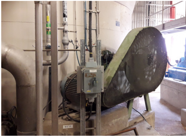
Old agitator installation
