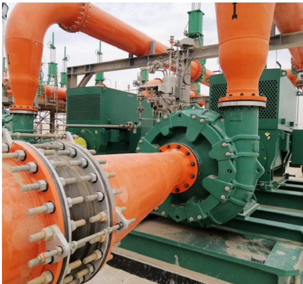
Heavy-duty slurry pump type EMW350MS at the site (2021).
