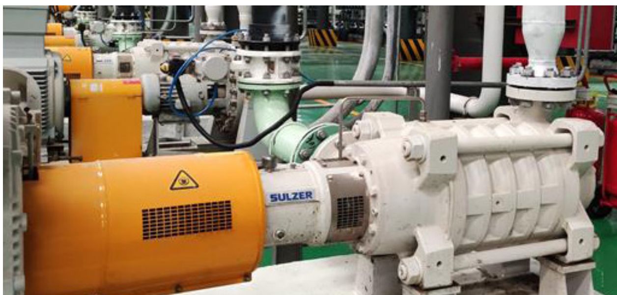
NF membrane feed pump
