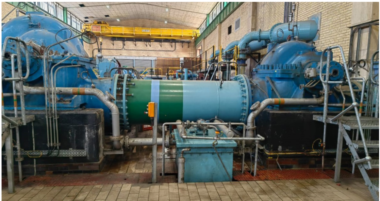
Sulzer is working with water utility companies to identify the pumps most set in need of refurbishment
