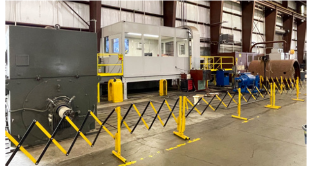
Multiple testing facilities from 460 volts to 13.8kv
