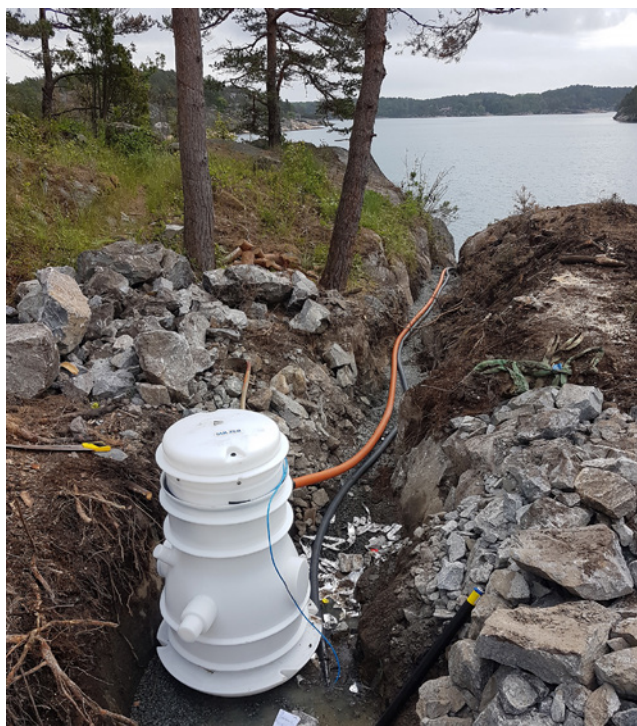
Flexible high-pressure pipes are easy to install in difficult ground and can even run over the bed of the fjord
