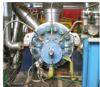
The retrofitted installation
