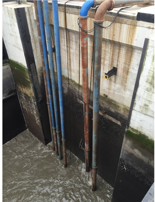
Rental pumps in the lock chamber: parallel installation of six flange pipes
