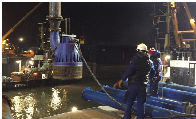
Rental pump connected to steel pipe DN 350 with flange
