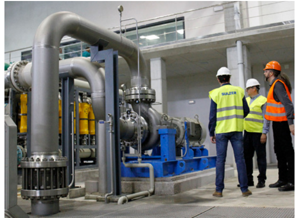
16 ERD booster pumps driven with variable speed drive support the efficient operation
