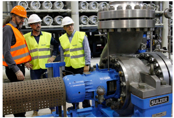
All the pumps use corrosion resistant super duplex stainless steel.
