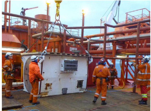
Engineers onboard an offshore platform for the safe commissioning of a repaired HV motor
