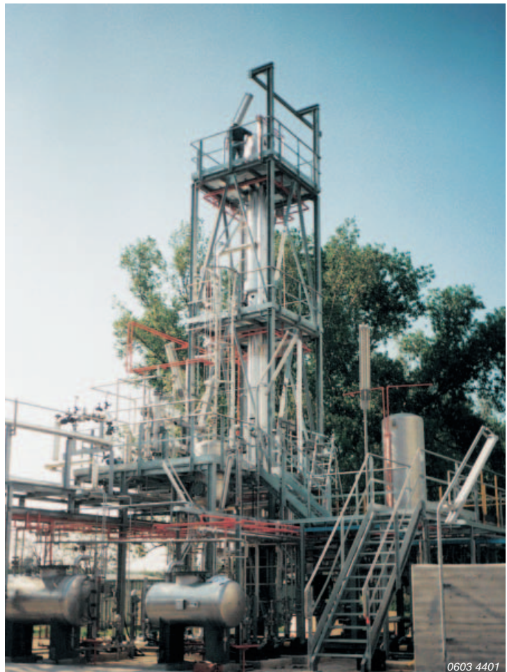
Distillation and vapor permeation unit
