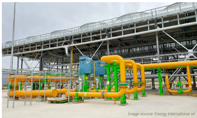
Sulzer's main feed pumps installed in a Binary Cycle Geothermal Power plant.
