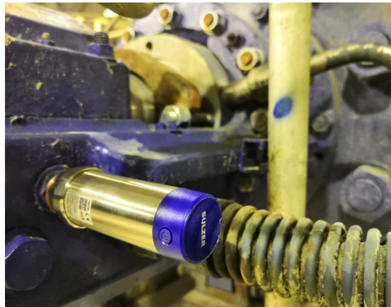
Sulzer Sense installation at a customer site.
