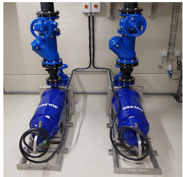
The XFP pumps working in a duty/standby arrangement, give the station a capacity of 25 liters per second.
