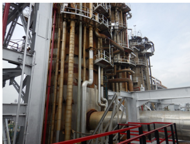
Radial feed inlet nozzle after revamp
