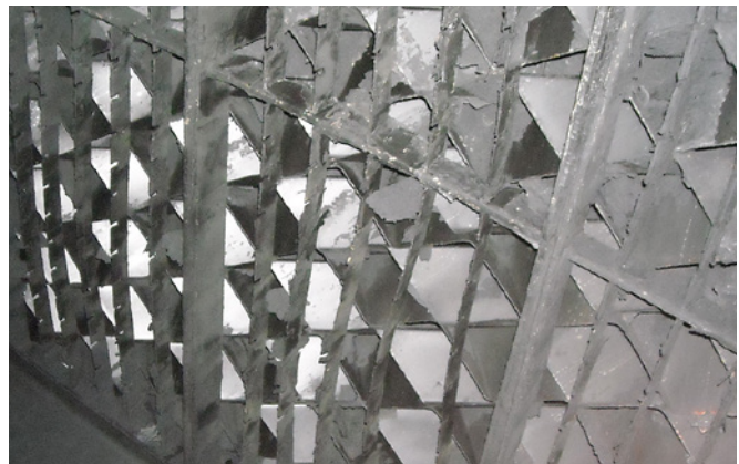
Mellagrid high-performance structured grid after 3 years operation, only small amount of coke at the bottom of the bed, washed in place and reused
