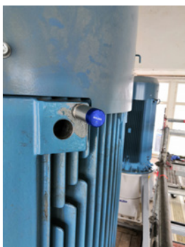
Sulzer Sense monitors the condition of two vertical pumps and motors.
