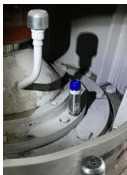
The sensors are installed in the bearings of the monitored equipment.
