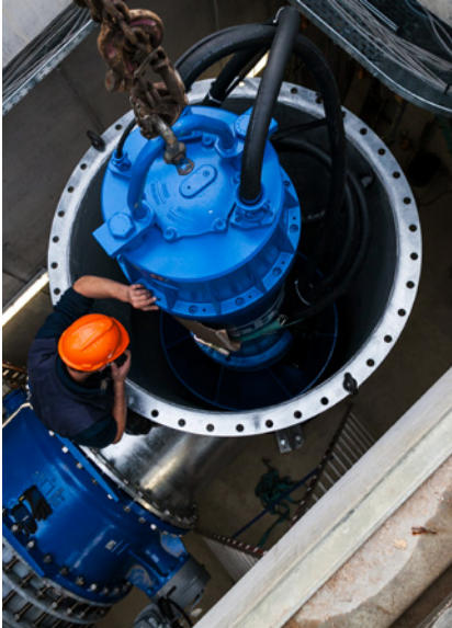
Installation of a vertical submersible propeller pump from Sulzer in a steel riser pipe in size DN 1600
