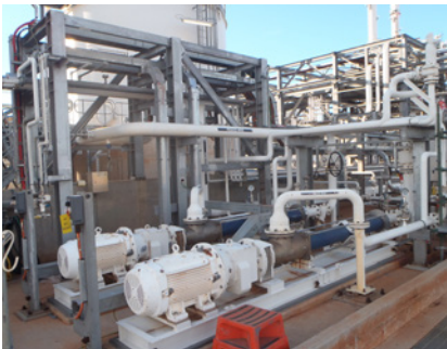
Existing Progressive Cavity Pumps
